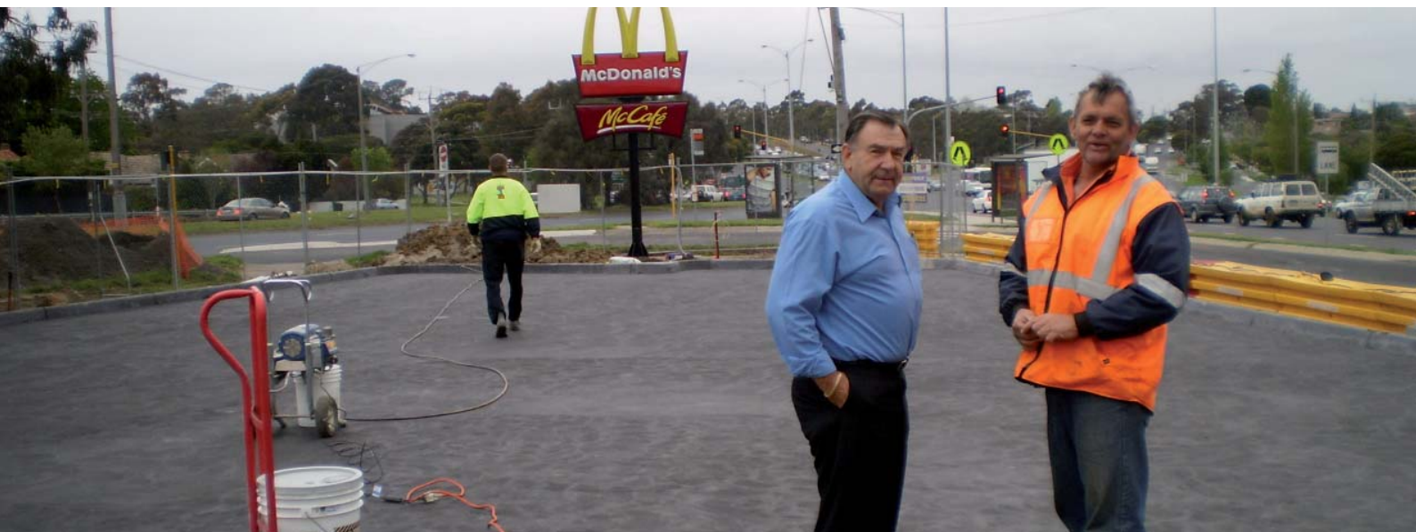
Terry Lucas and Paul Mickus, Site Manager for Lansky Constructions at North Road McDonalds car park only hours after placement by the concreters, watching the commencement of the Densi-Proof application.
