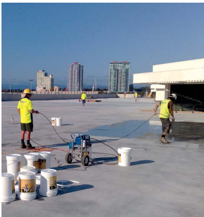
The application of Densi-Proof saves time and money and allows site access to other trades within one hour.
