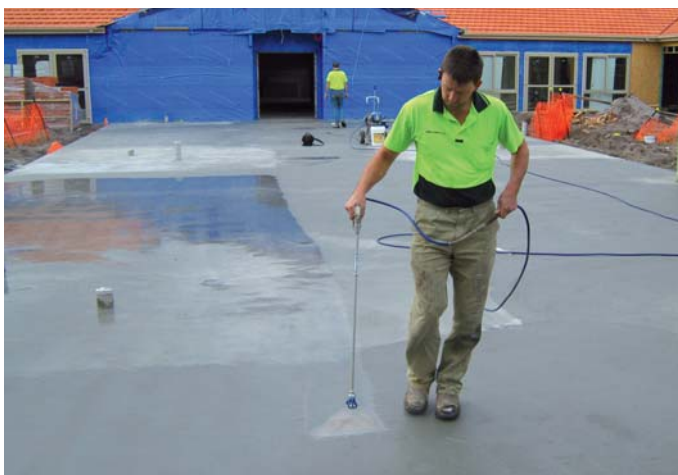
Ken Arnott of Kenbar Floors applies Protect Crete Densi-Proof at time of pour as cure and moisture barrier.
