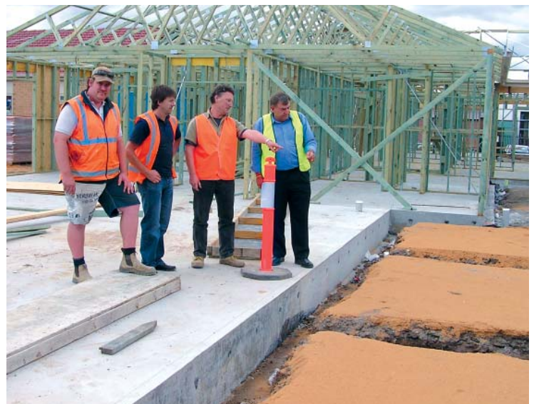
Dave Sutton, Ken Arnott, Peter Rawlins and Terry Lucas, on slabs already treated and protected, inspecting the next pour site.
